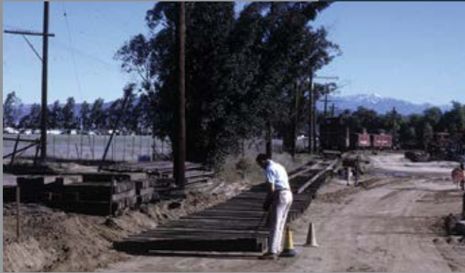
Figure 19-01: Track laying on the north side of the Loop approaches the northwest corner. The view is to the east. (SCRM Archives/Jim Walker photo)
