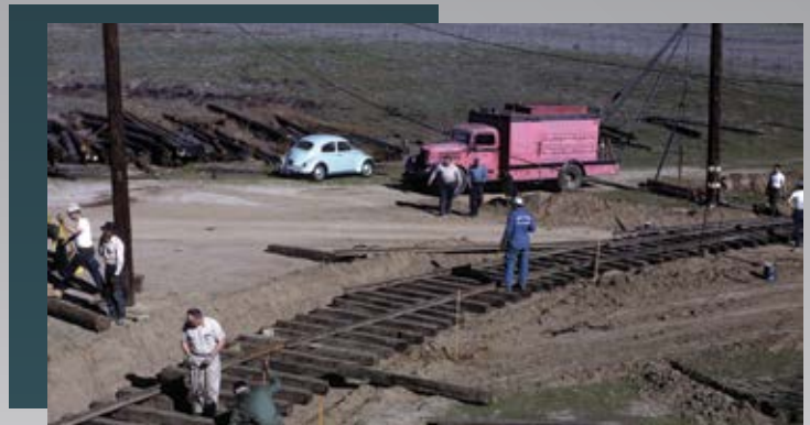
Figure 19-02: Track laying around the northwest corner of the Loop approaches the new bookstore-station building. Alpine Drive comes in from the left. (SCRM Archives/Jim Walker Photo)
